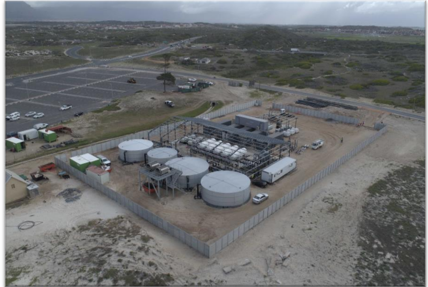
Strandfontein Temporary Desalination Plant (7 MLD)
