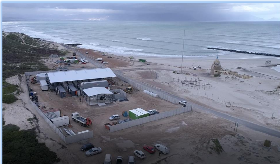
Monwabisi Temporary Desalination Plant (7 MLD)
